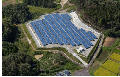
S-02 CS Isa-shi Power Plant 0.9MW
