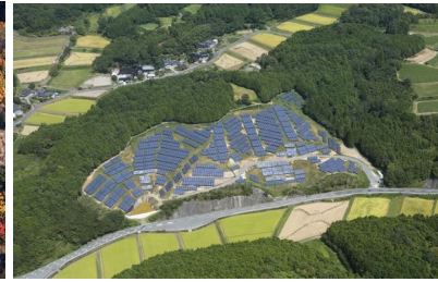
S-15 CS Tsuyama-shi Power Plant 2.0MW
