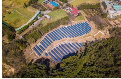
S-18 CS Takayama-shi Power Plant 1.0MW
