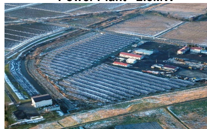
S-22 CS Ishikari Shinshinotsu-mura Power Plant 2.3MW
