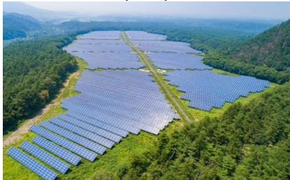
S-17 CS Daisen-cho Power Plant (A&B) 27.3MW
