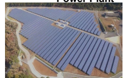
S-09 CS Ashikita-machi Power Plant
