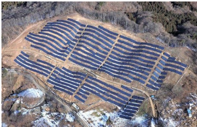
S-11 CS Minano-machi Power Plant 2.4MW
