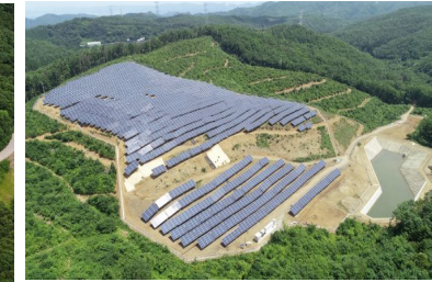
S-20 CS Marumori-machi Power Plant 2.2MW
