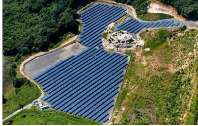
S-07 CS Kasama-shi Dai-ni Power Plant 2.1MW
