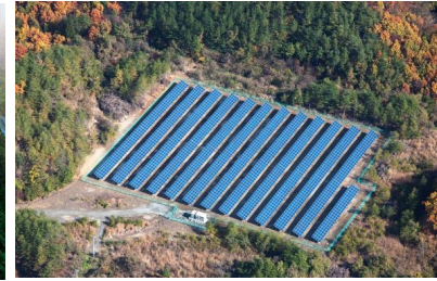
S-14 CS Koriyama-shi Power Plant 0.6MW
