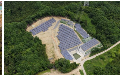
S-19 CS Misato-machi Power Plant 1.1MW
