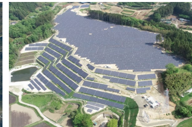
S-25 CS Ogawara-machi Power Plant 7.5MW
