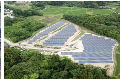
S-23 CS Osaki-shi Kejonuma Power Plant 0.9MW
