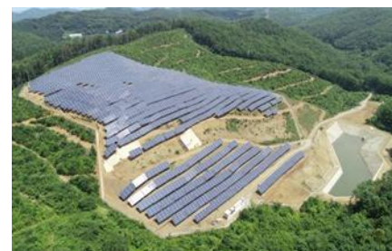
S-20 CS Marumori-machi Power Plant 2.2MW
