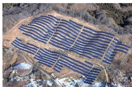
S-11 CS Minano-machi Power Plant 2.4MW
