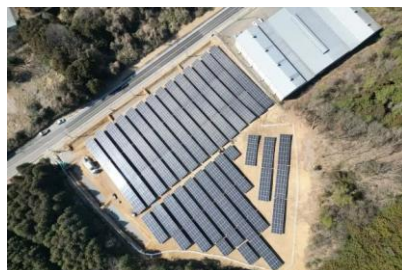
S-34 CS Sakura-shi Kitsuregawa Power Plant 1.2MW
