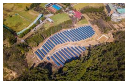
S-18 CS Takayama-shi Power Plant 1.0MW
