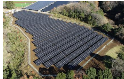
S-35 CS Tsukuba-shi Takamihara Power Plant 1.1MW
