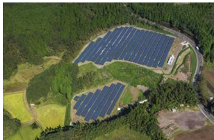
S-05 CS Yusui-cho Power Plant 1.7MW
