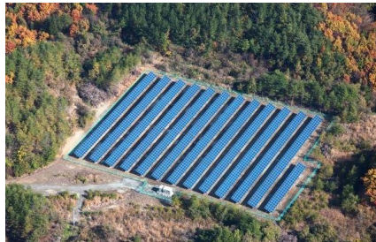
S-14 CS Koriyama-shi Power Plant 0.6MW
