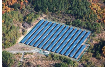
S-14 CS Koriyama-shi Power Plant 0.6MW
