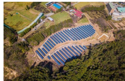
S-18 CS Takayama-shi Power Plant 1.0MW
