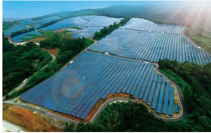
S-13 CS Mashiki-machi Power Plant 47.7MW
