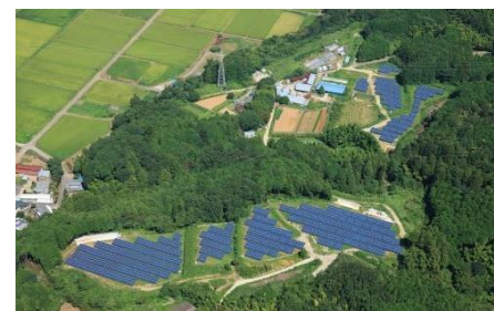
S-12 CS Kannami-cho Power Plant 1.3MW
