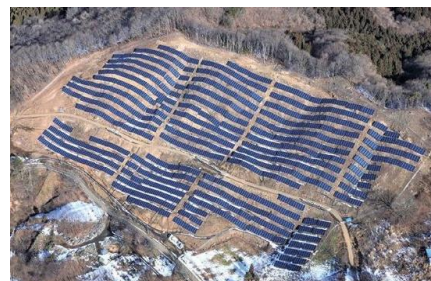
S-11 CS Minano-machi Power Plant 2.4MW
