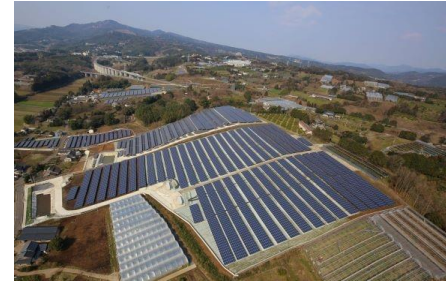
S-08 CS Hiji-machi Power Plant 2.6MW
