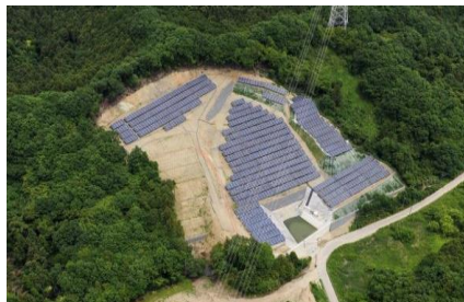
S-19 CS Misato-machi Power Plant 1.1MW
